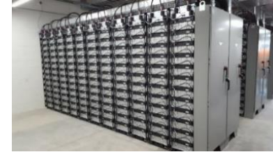
AltaGas 80MWh Li-Ion battery installation: http://www.marketwired.com/press-release/altagas-celebrates-opening-of-north-americas-largest-battery-storage-facility-tsx-ala-2191585.htm
