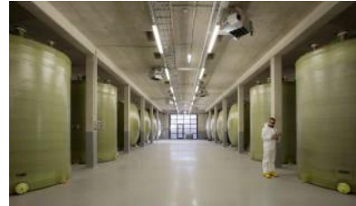
Fraunhofer ICT 20MWh Redox Flow Battery: https://www.ict.fraunhofer.de/de/komp/ae/rfb.html
