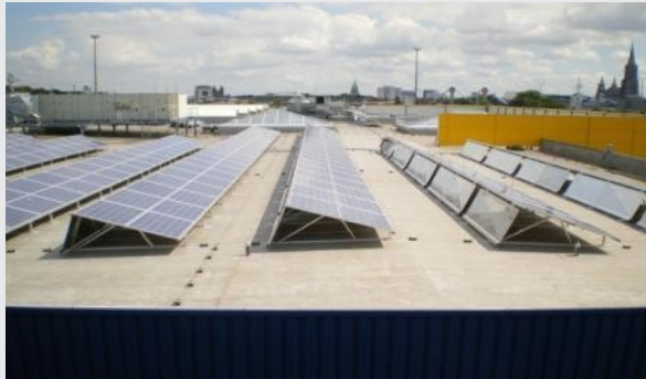
IKEA Ulm – 250 kWp
