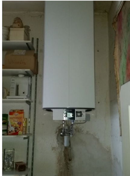
Boiler ca. 2 KW
